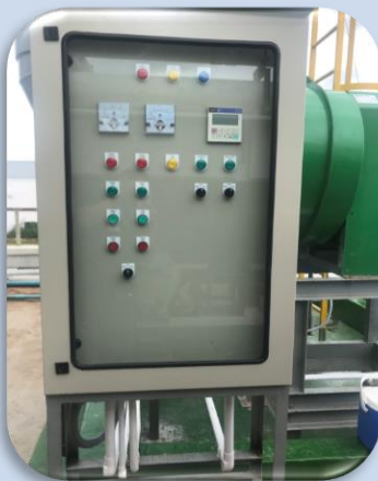
Electrical Control System
