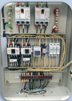
Electrical Control System
